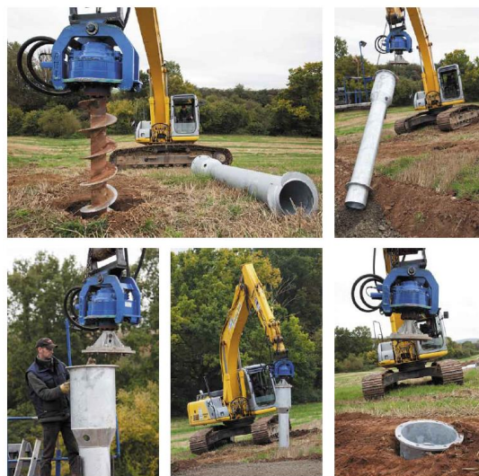
▲ Installing a screw foundation for a dual-axis tracking system (Dager-Traker) at Am Peterswald PV park in Germany. Bftec GmbH pre-drills the ground at the site and then the foundation is installed. The foundation's unusual form, which consists of a smooth side wall with a coil at the bottom (if necessary, two coils), guarantees a firm grip. The foundation can rotate in the ground without displacing or loosening the surrounding earth.
